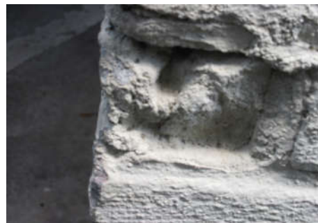
Some damaged brick found throughout.
