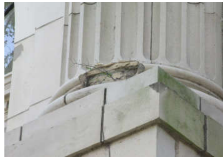
Terra cotta damage found throughout.
