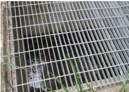
We are uncertain if these ventilation holes are intended to hold water.
