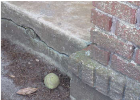
Cottage front stoop is damaged.
