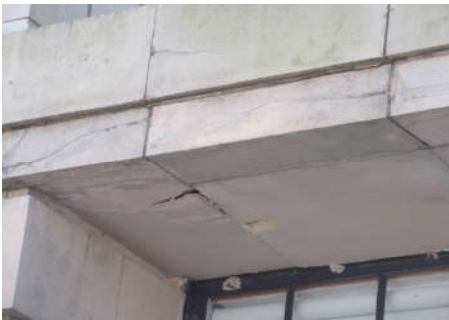
Terra cotta damage found throughout.
