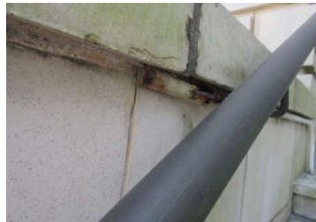
Exterior conduit needs to be replaced.
