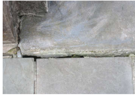
There appears to be void that should be filled.
