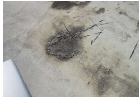
Evidence of standing water.
