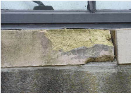
Some damaged brick found throughout.
