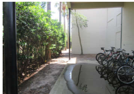
Standing water is a minor issue, but will like cause the surface of concrete to deteriorate faster.
