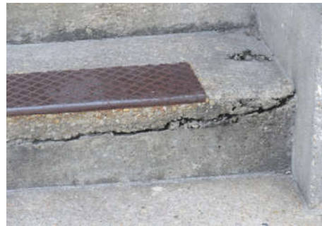
Annex step is damaged.
