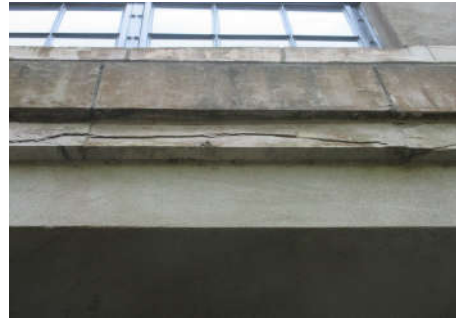
Terra cotta damage found throughout.
