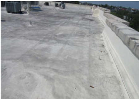
Roof is assumed to be replaced after the report is issued, but before the reserve window.
