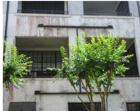
Building surface should be cleaned.
