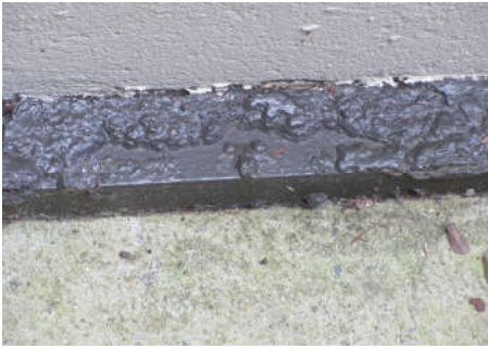
Rust has formed on the exterior metal stairs.
