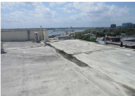
Evidence of standing water.
