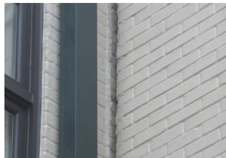
An engineer needs to review the walls abutting the exterior metal stairs at the annex.
