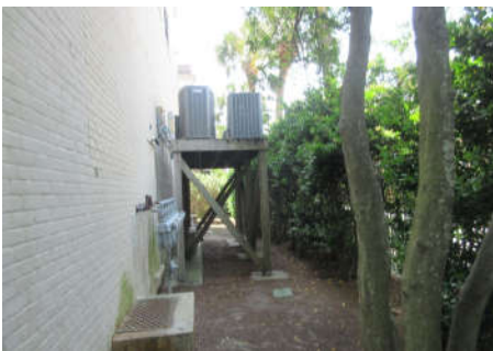
The HVAC stand feels secure, but should be replaced or reviewed by engineer due to its age.
