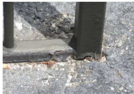
This railing will fail earlier than intended due to being embedded in this manner.
