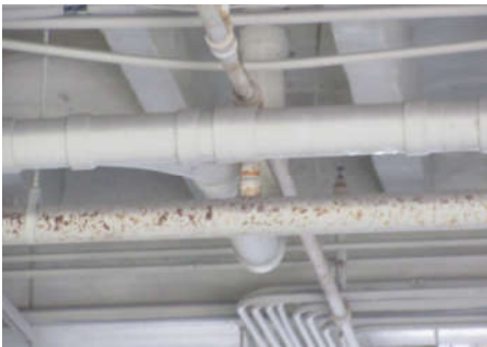
Exposed pipes in the garage should be repainted.
