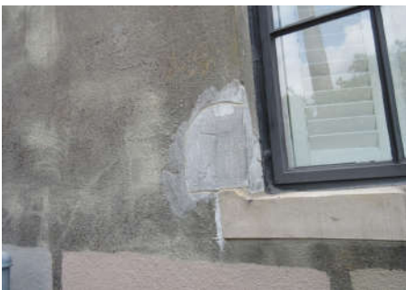
Stucco repairs and painting should be performed.
