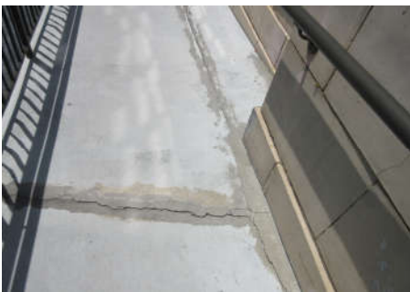
Cracking found at the ADA ramp.
