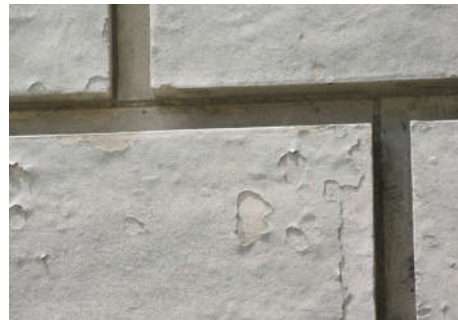
The terra cotta surface should be recoated.
