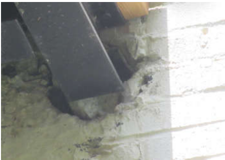
Engineer should review the homeowner deck attachments. This may not be properly flashed.
