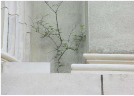
Remove debris build up to prevent organic growth.
