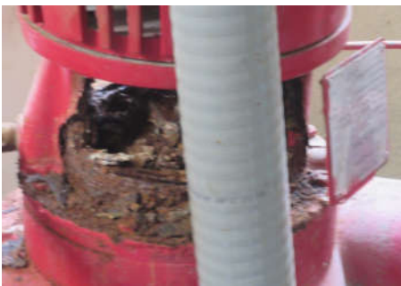
Sprinkler motor should be replaced.
