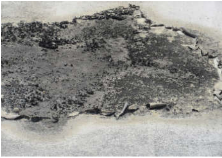
Roof surface is delaminating.
