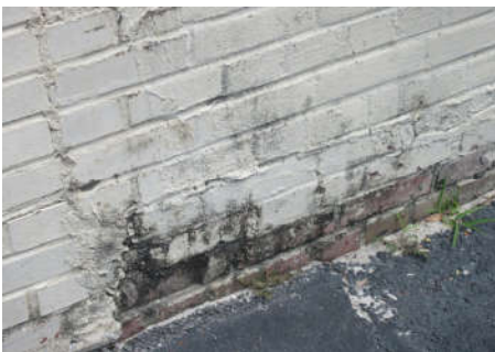
Some damaged brick found throughout.
