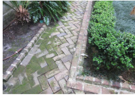
The brick pavers need to be reset.
