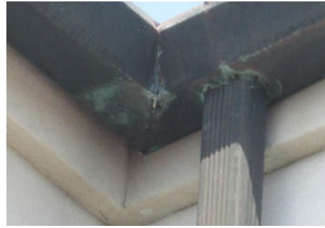
Main gutter system appears to be leaking.
