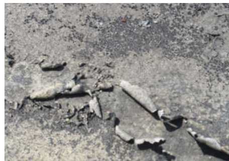
Roof surface is delaminating.
