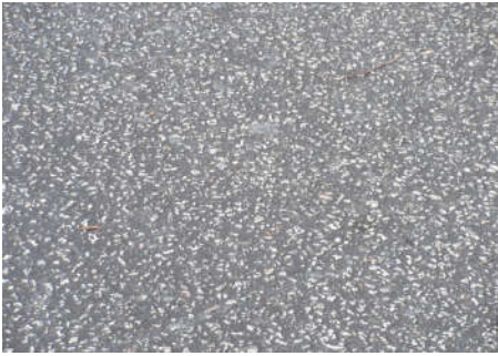
Fine aggregates have eroded from the surface, accelerating the parking lot's decline.
