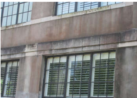
Building surface should be cleaned.
