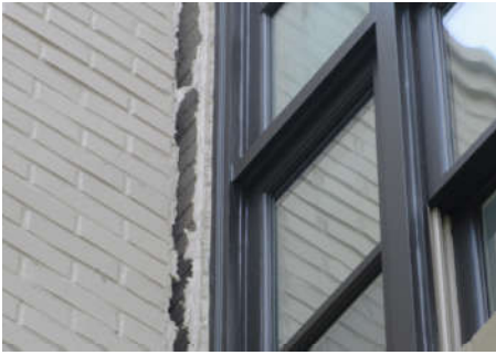
An engineer needs to review the walls abutting the exterior metal stairs at the annex.
