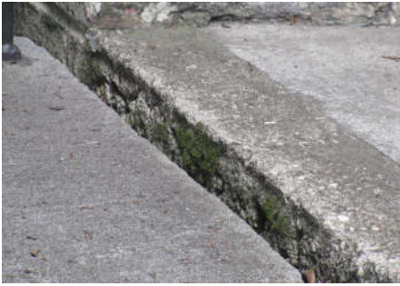
Section of concrete at garage has sunk, causing a tripping hazard.
