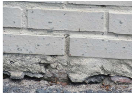
Mortar deterioration along the bottom of wall should be addressed intermittently.
