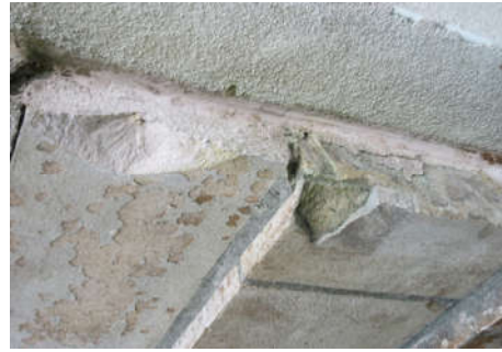
Terra cotta damage.
