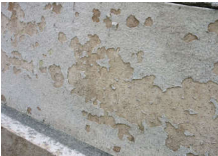
The terra cotta surface should be recoated.
