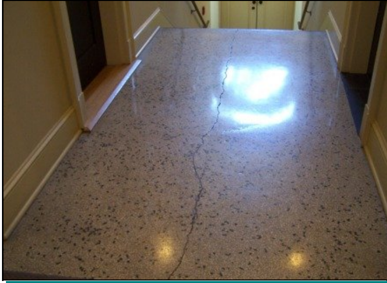
Terrazzo floors - Note cracks Fund honing of terrazzo through operating budget
