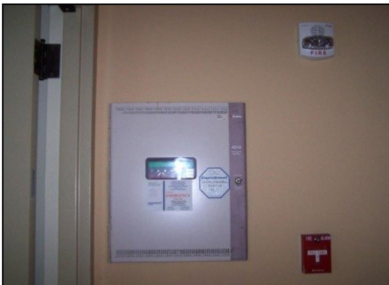
Fire detection system devices
