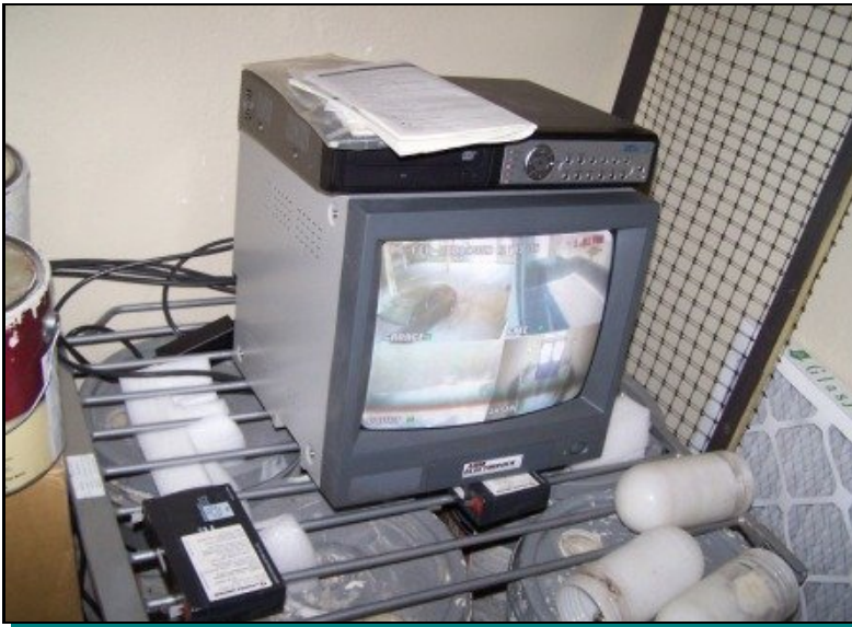
Security system monitoring equipment
