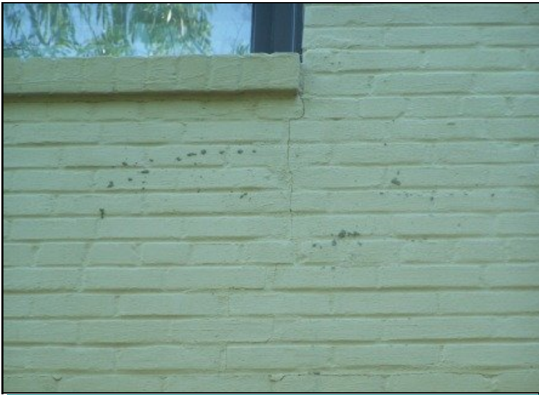
Masonry walls - Note cracks
