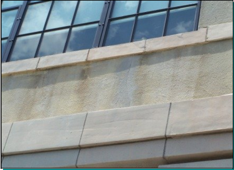
Stucco walls - Note cracks and discoloration
