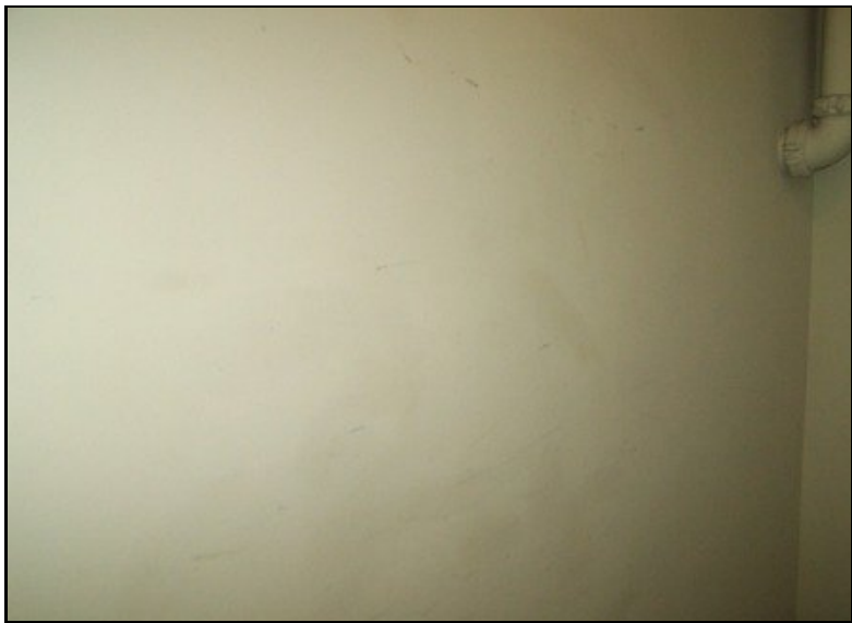
Paint finish - Note scuff marks
