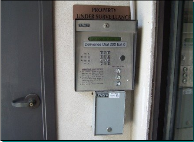
Typical intercom panel
