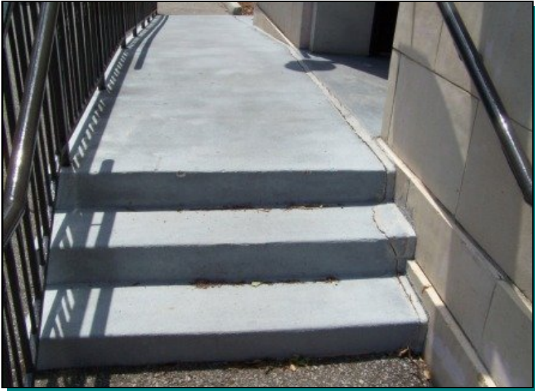
Concrete flatwork - Note concrete cracks
