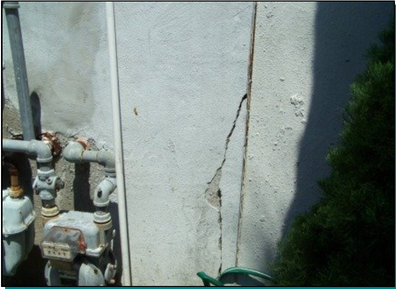
Stucco walls - Note cracks
