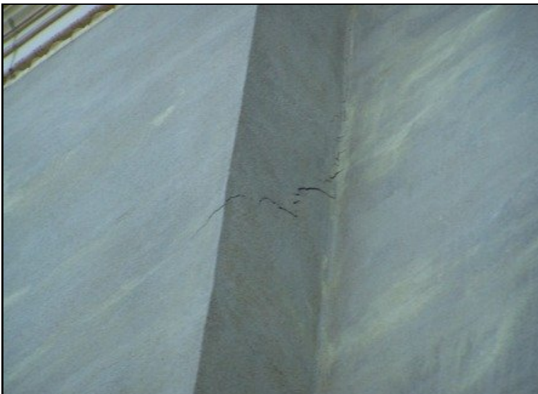
Stucco walls - Note cracks
