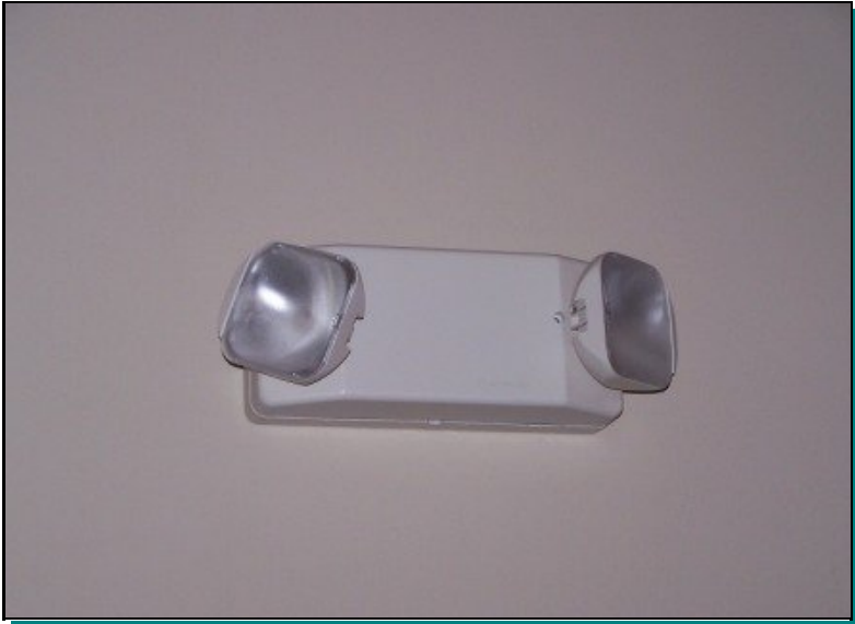
Typical emergency light fixture
