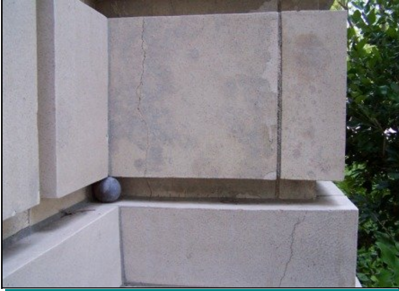
Masonry walls - Note finish deterioration and cracks
