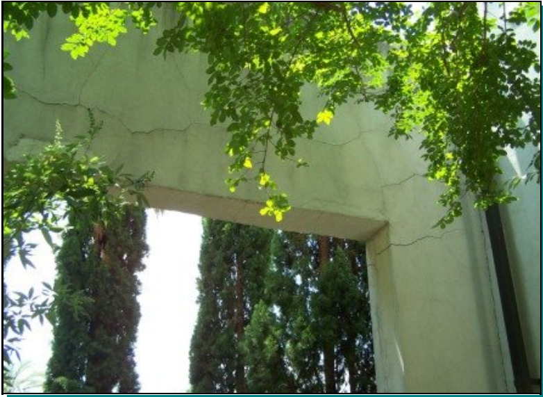
Stucco walls - Note cracks
